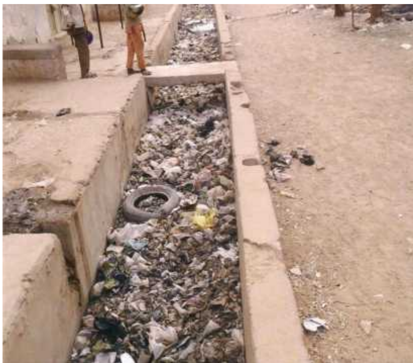
Plate 1: A gutter at Kofar Kaura, Katsina City. Source: Field work, 2016
